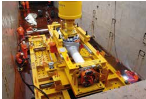
Subsea Riser Positioning
